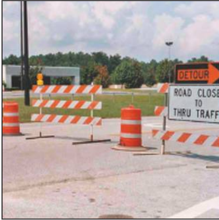
Shannon Parkway cannot be used by MARTA buses due to structural problems
